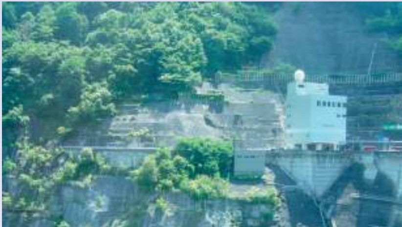
Concreting a mountainside in the Japanese Alps, by a hydroelectric dam. Raphaël Languillon-Aussel, August 2012
